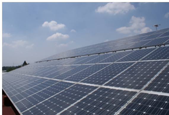
Fig. 1. Shows part of 60 kWp PV module array in CINVESTAV, Mexico City.
