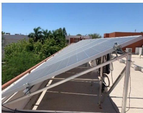
a) Photovoltaic system.
